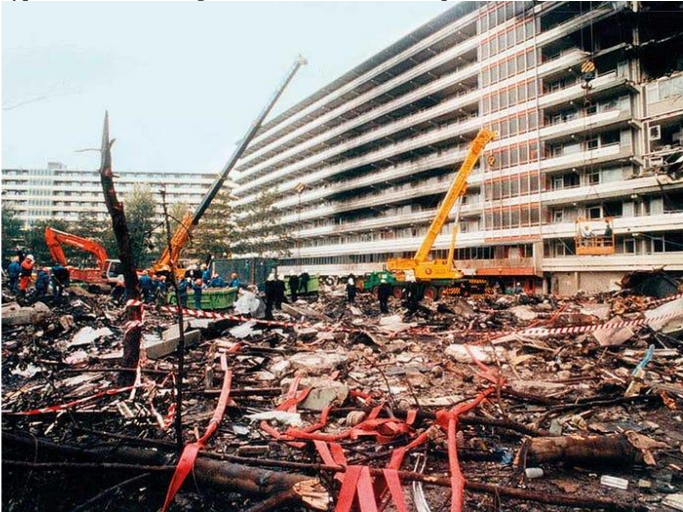
Cranes work to clear debris from in front of the apartment buildings. (Gulf News)
